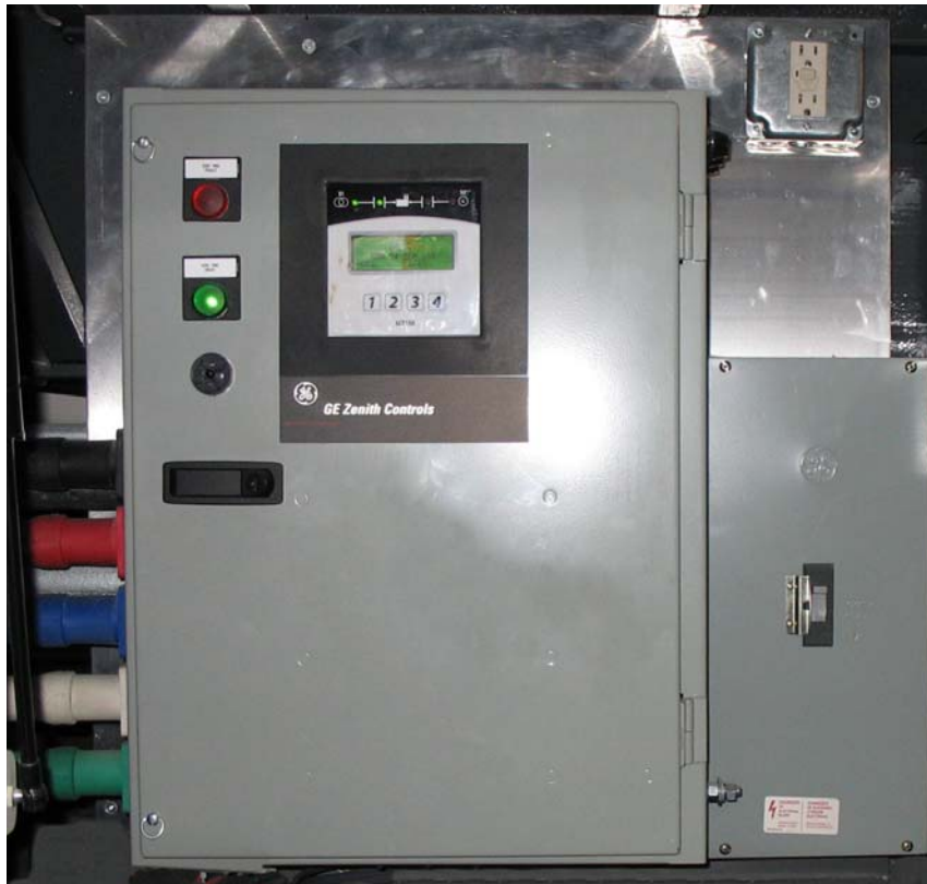
Figure 10: Automatic Transfer Switch (ATS)
