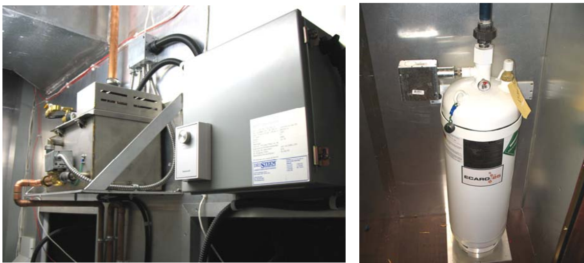
Figure 17: Mechanical Room Overall
