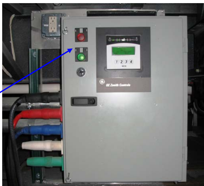
Figure 29: 220V AC Phase Power Monitor
