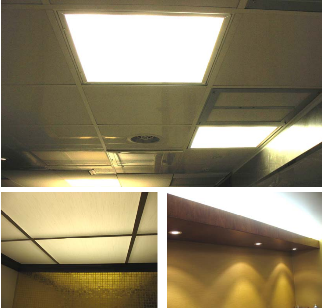
Figure 41: Interior Overall Lighting
