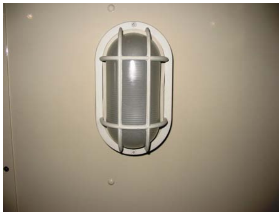
Figure 40: Entry Door Lighting
