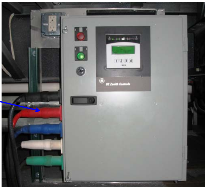
Trailer Underbody Power Connections
