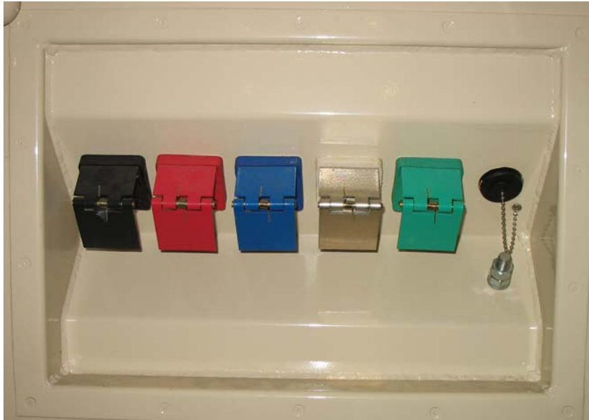
Figure 14: Generator Cam-lock Connectors
