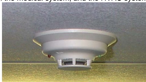
Figure 4: Smoke / Carbon Monoxide Detector
