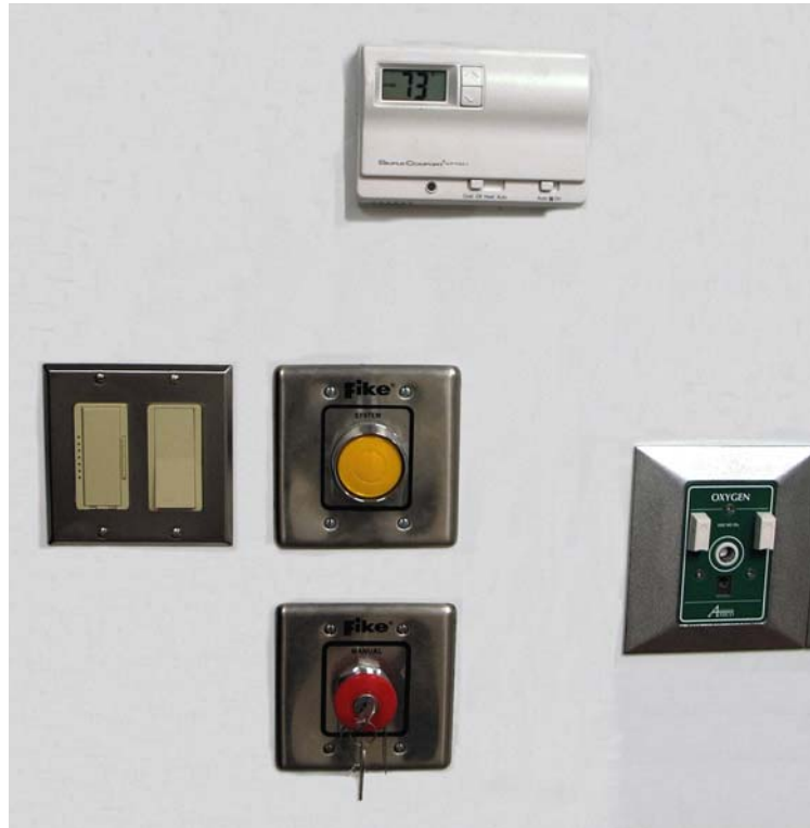
Figure 18: Mobile Unit Controls
