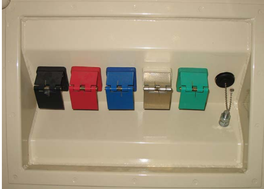
Figure 25: Generator Power Cable to Trailer Cam-lock Connectors
