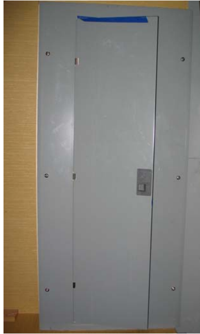
Figure 27: 220/127V AC Electrical Panels
