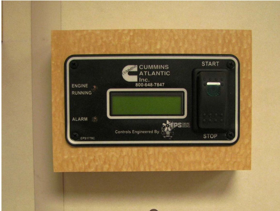
Figure 29: Generator Remote Start / Stop Switch
