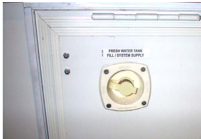
Figure 33: Fresh Water Connection
