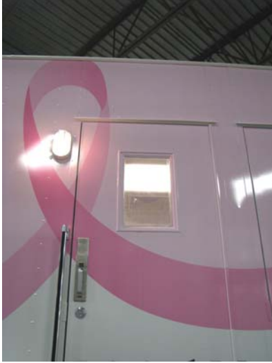
Staff Door Entry Light
