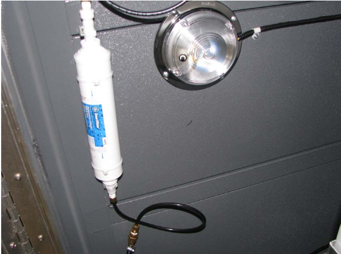
Figure 35: Humidifier Water Sediment Filter
