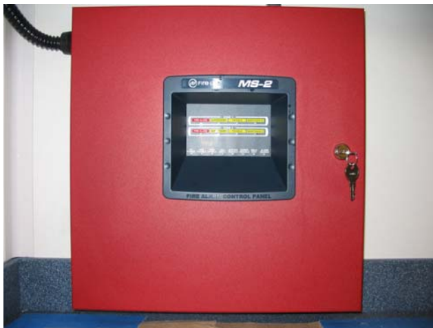
Figure 19: Fire Alarm Control Panel
