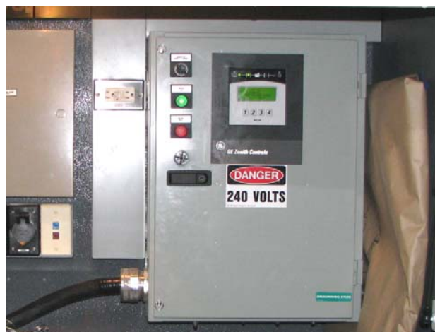
Figure 22: Automatic Transfer Switch (ATS)
