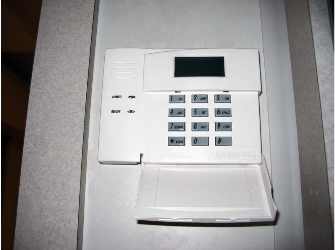
Figure 39: Intrusion Alarm Keypad
