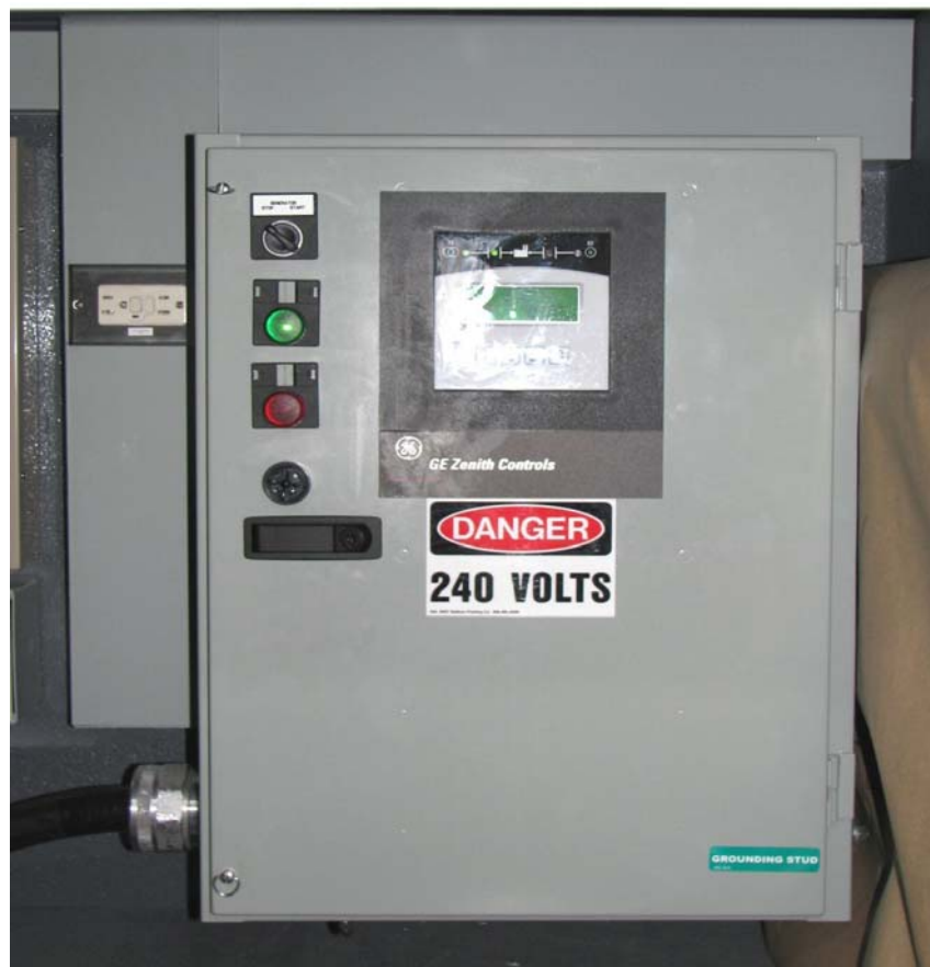
Figure 28: Automatic Transfer Switch (ATS)
