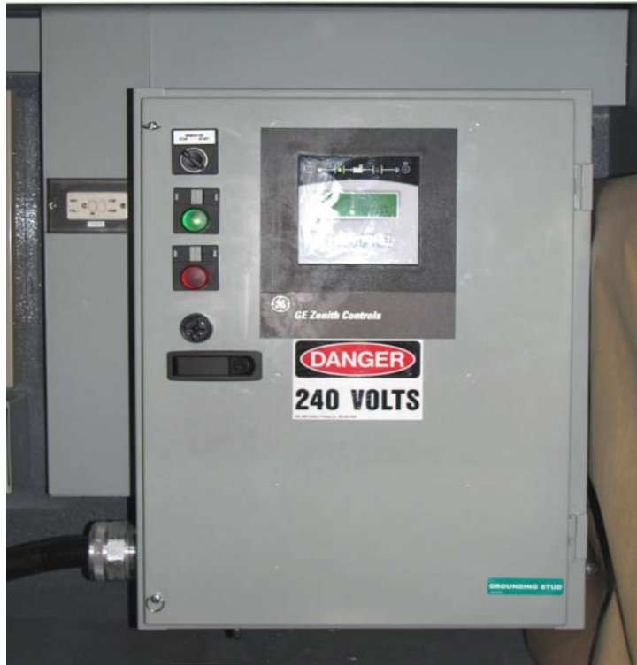
Figure 23: 240V AC Electrical Panel Automatic Transfer Switch
