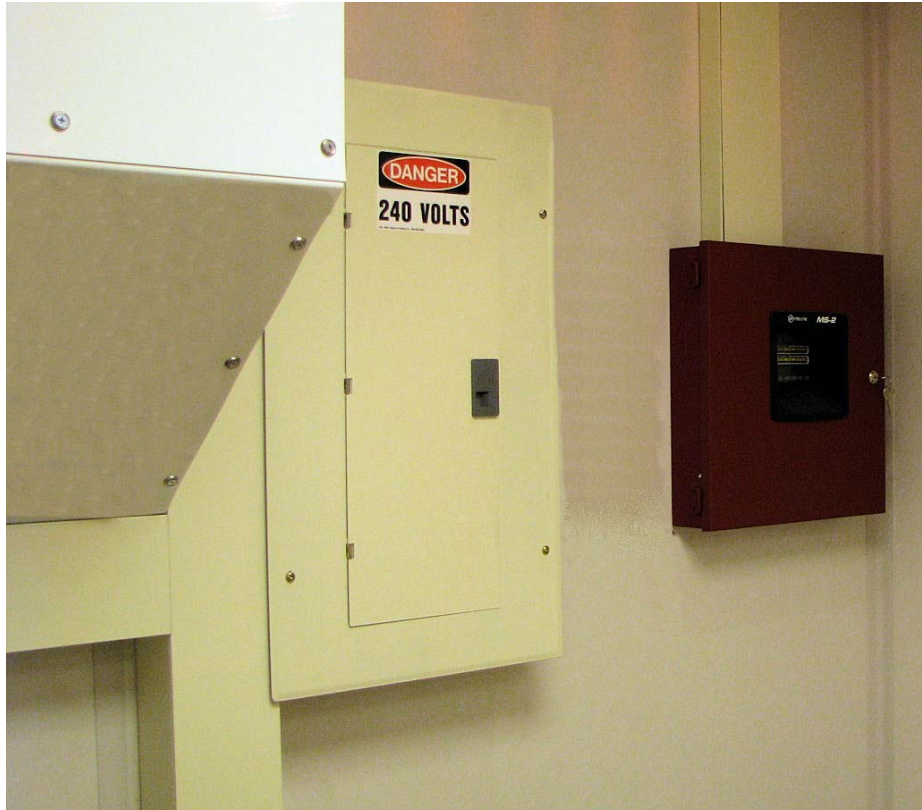
Figure 24: 120/240V AC Electrical Panel
