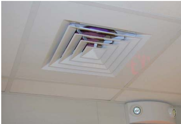
HVAC Vents Discharge
