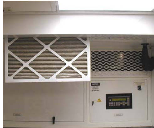
HVAC Filter Access
