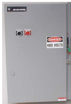
Figure 36: A1 Electrical Panel
