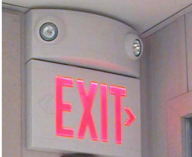
Figure 54: Emergency Dual Beam Lighting
