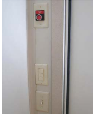
Control Room Lighting and E-Stop
