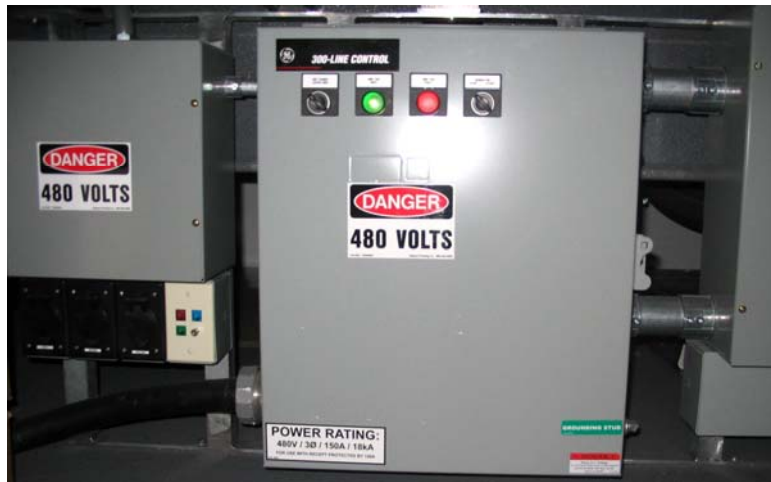
Figure 9: Power Supply Control Panel
