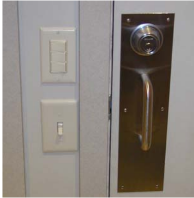
Scan Room Lighting
