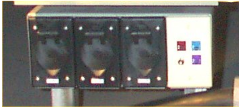
Figure 17: Phone & Data Line Connections
