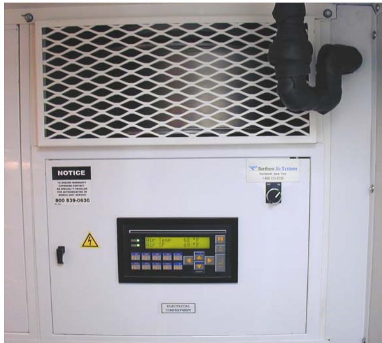
Figure 45: A/C / Chiller Control Panel
