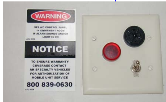
Air Conditioning Trouble Light & Alarm Figure 16 Mobile Unit Controls
