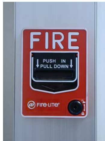
Figure 28: Fire Alarm Pull Station
