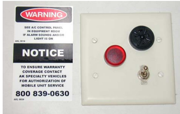
Figure 46: A/C / Chiller Alarm Panel
