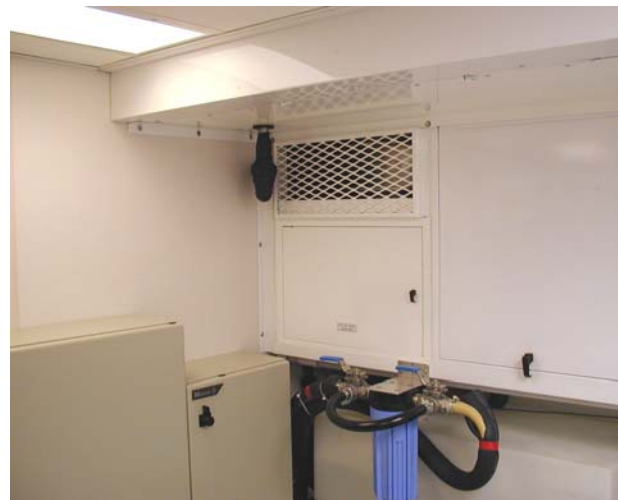
Figure 59: Equipment Room Lighting
