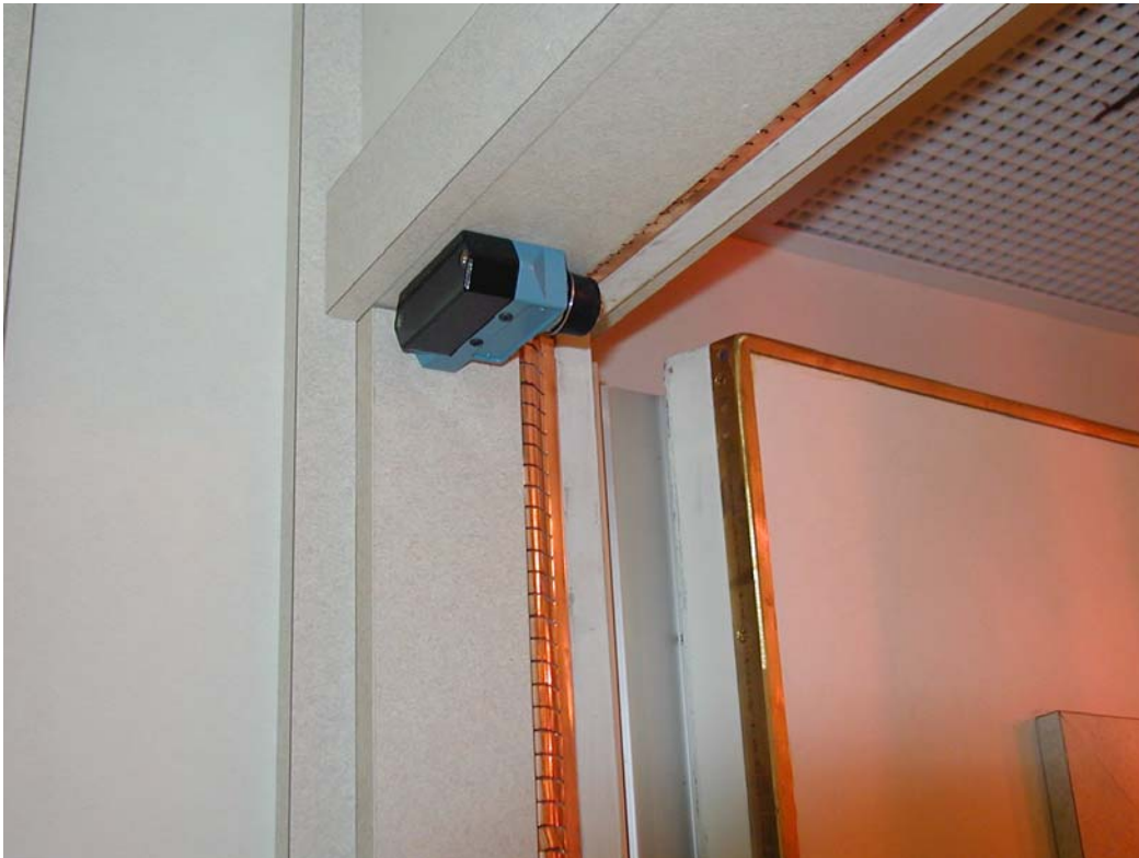
Close up of RF door trim
