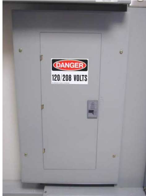
Figure 34: 208V AC Electrical Panel
