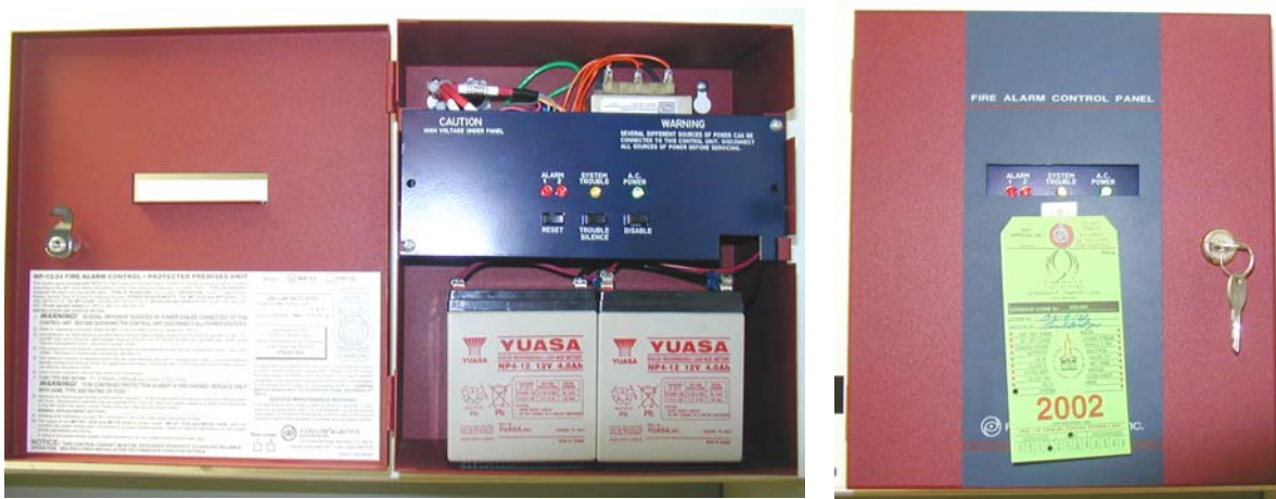
Figure 27: Fire Alarm Control Panel
