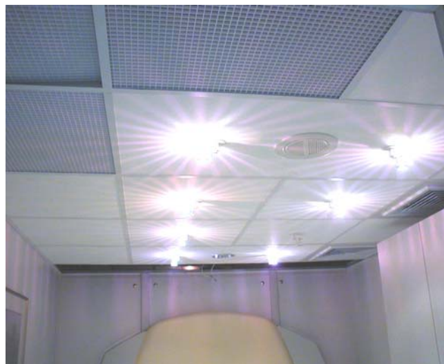
Figure 61: Scan Room Lighting
