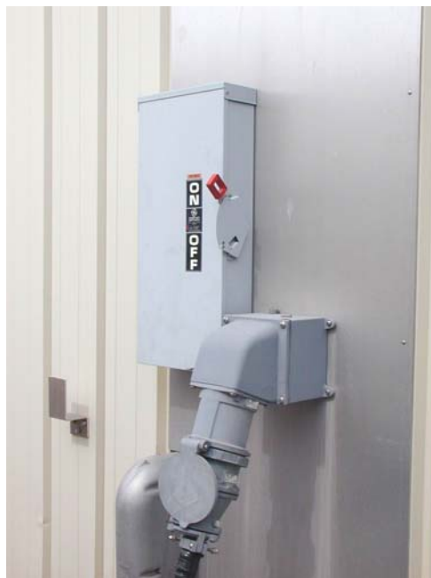
Figure 37: Shore Power Connection
