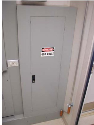
Figure 35: 480V AC Electrical Panel
