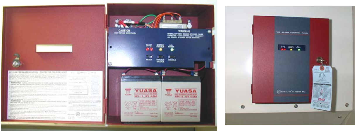
Figure 20: Fire Alarm Control Panel
