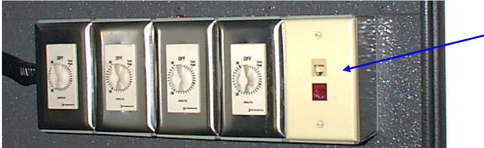
Figure 13: Phone & Data Line Connections
