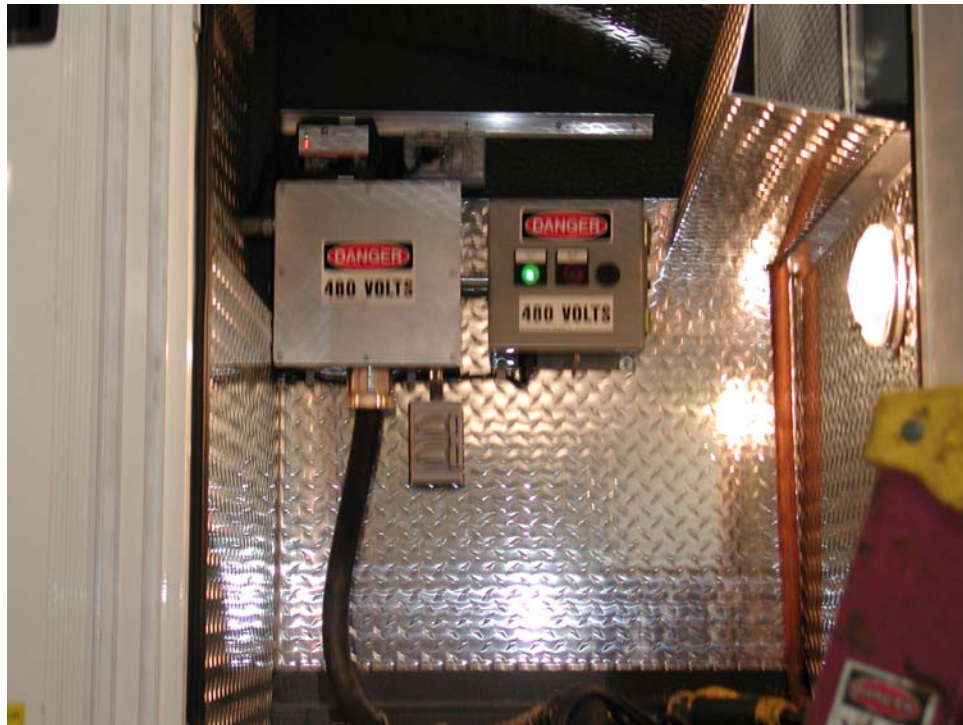
Figure 26: 480V AC Phase Power Monitor
