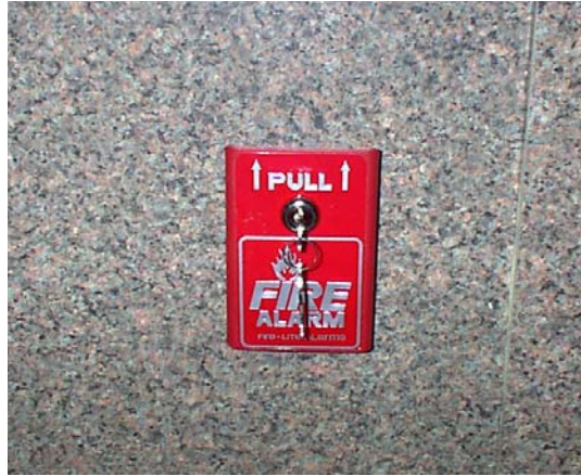
Figure 21: Fire Alarm Pull Station
