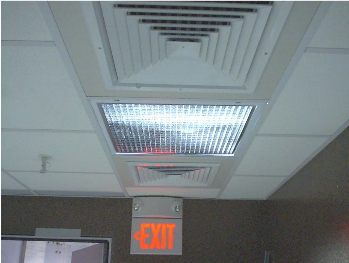
Figure 40: Interior Overall Lighting
